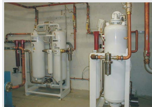
Installation in der Uniklinik in Innsbruck (4x ATM 37)
